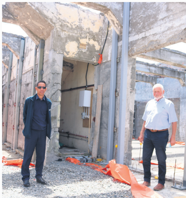
Council Chief Executive Kitea Tipuna and myself surveying the strengthening progress inside the former main street burnt-out building shell.
