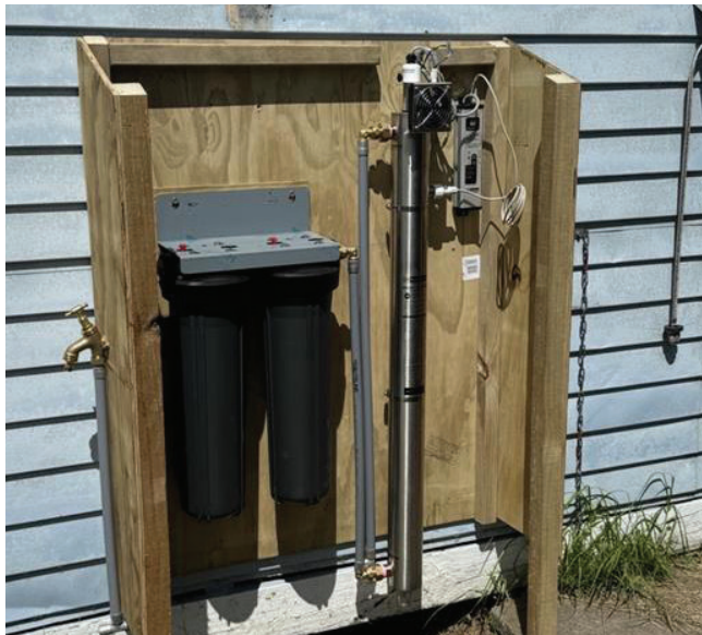
Installation of Nuhaka Rugby Club UV system.
