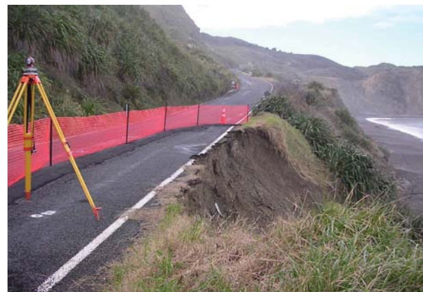
This drop-out at Black's Beach serves as an example of a major roading project requiring months of 'behind-the-scenes' work.
