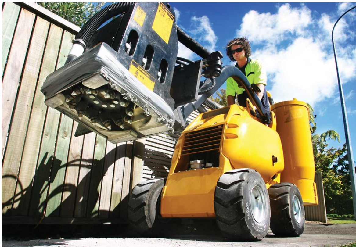
Driver John Hindle takes the concrete grinder through its paces. Photo courtesy of Manawatu Standard Ltd.
